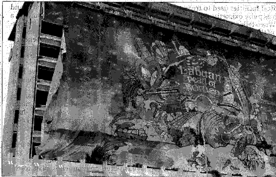
The damaged canvas billboard.
