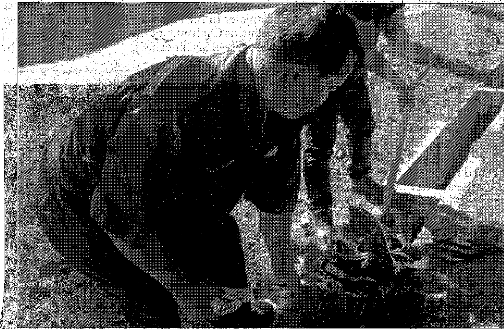
Workers clearing the clogged drain. Clearing the stagnant water at the shophouse.
